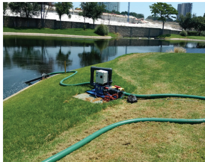
Installation of the Moleaer nanobubble generator does not require submersion into the pond.
