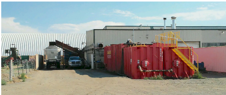
Photo of aeration cells at slaughter house
