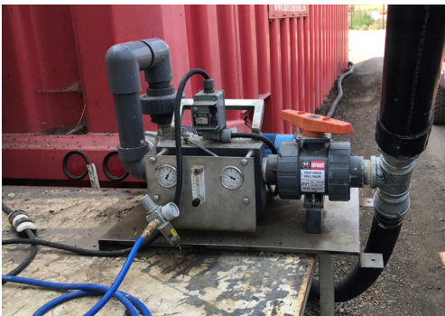
200 GPM XTB Nanobubble Generator installed at Idaho slaughterhouse
