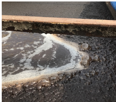
Sludge flotation in aeration cell #3 after installation of XTB
